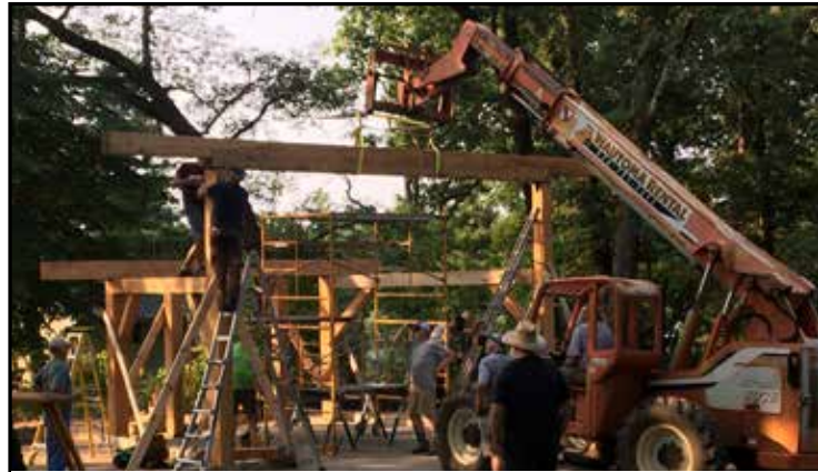
Rafters of Douglas Fir, columns & beams milled from repurposed utility poles, roof deck of local red pine.
