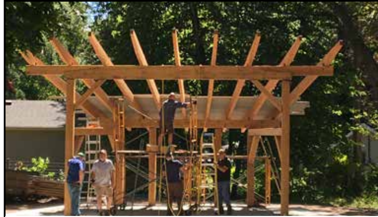
Led by Dave Erickson, this hard-working crew was able to complete most of the work in under a month!
