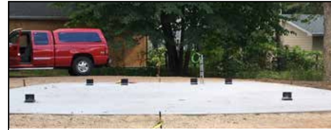
The concrete base was poured August 4 and the base plates were installed August 23.
